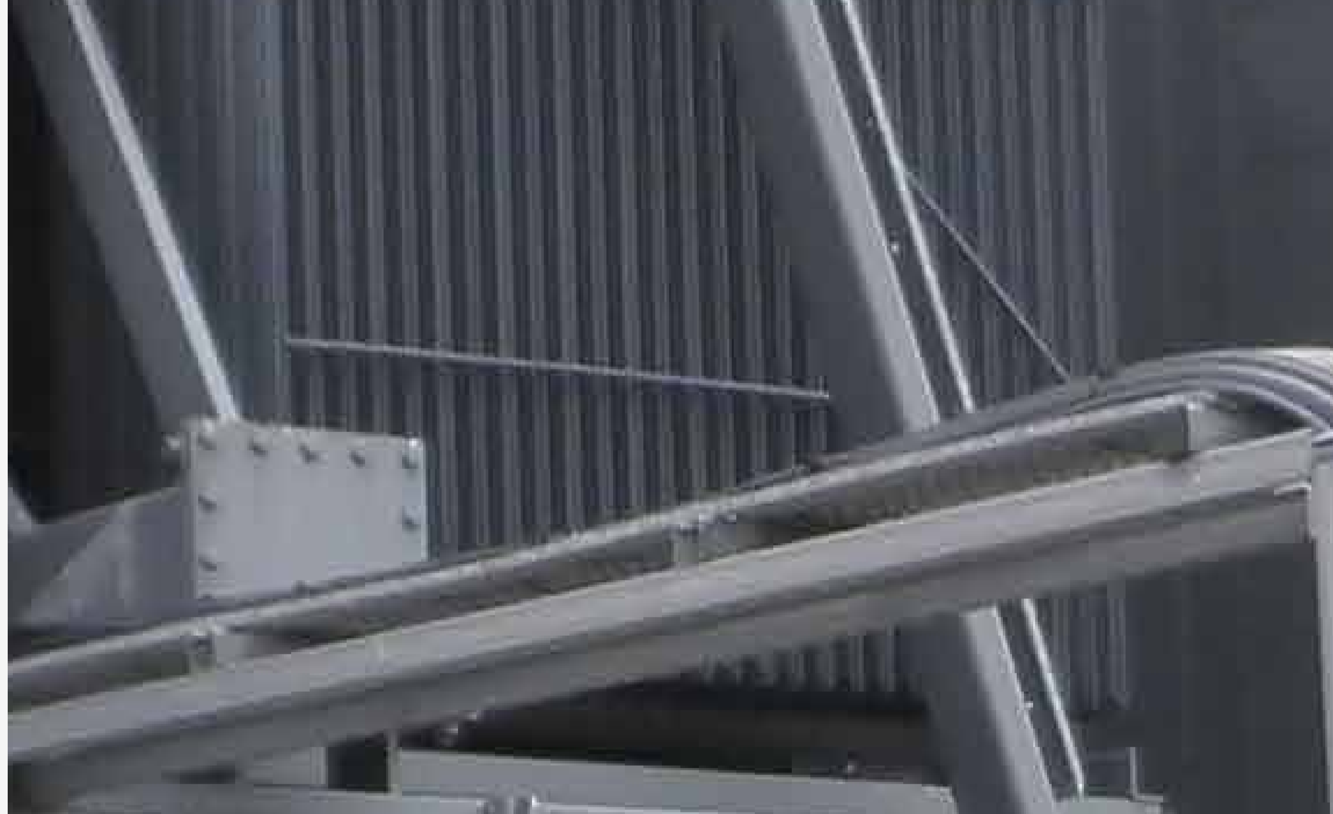
Image of typical (large 400kV) power transformer
